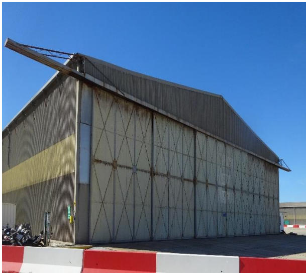
T2 Hangar – old doors
